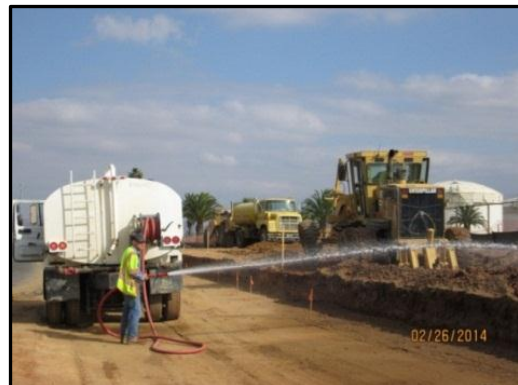
Pictured above are ongoing grading operations along Cactus Avenue necessary for the addition of the third lane from the I-215 eastbound off-ramp to Veterans Way.
