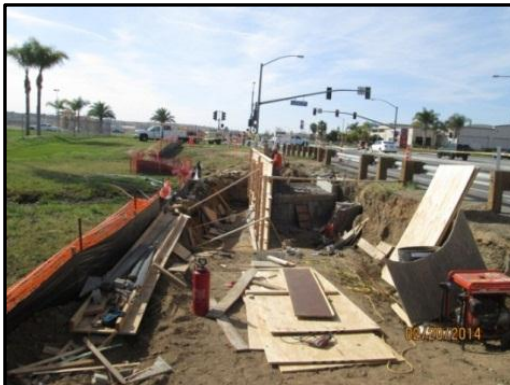
Pictured above is the construction of a culvert drain system that will be located under the new third lane on the south side of Cactus Avenue, east of Elsworth Street.
