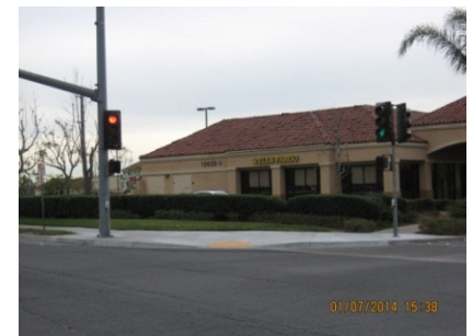
AFTER Installation of ADA Compliant Access Ramps & Pedestrian Push Buttons at the Southeast Corner of Centerpointe Drive and Centerpointe Plaza
